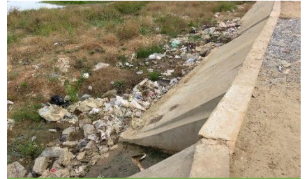
Rubbish at the creek near 2 nd street
