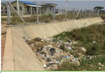
Rubbish at the creek near Main Road C
