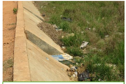
Rubbish at the creek near 6 th Street
